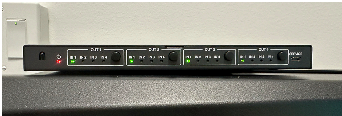
Figure 1: Front of the switcher. View shows input settings for using the TEACHER station. Press the round black button in each output section to switch to different inputs.
